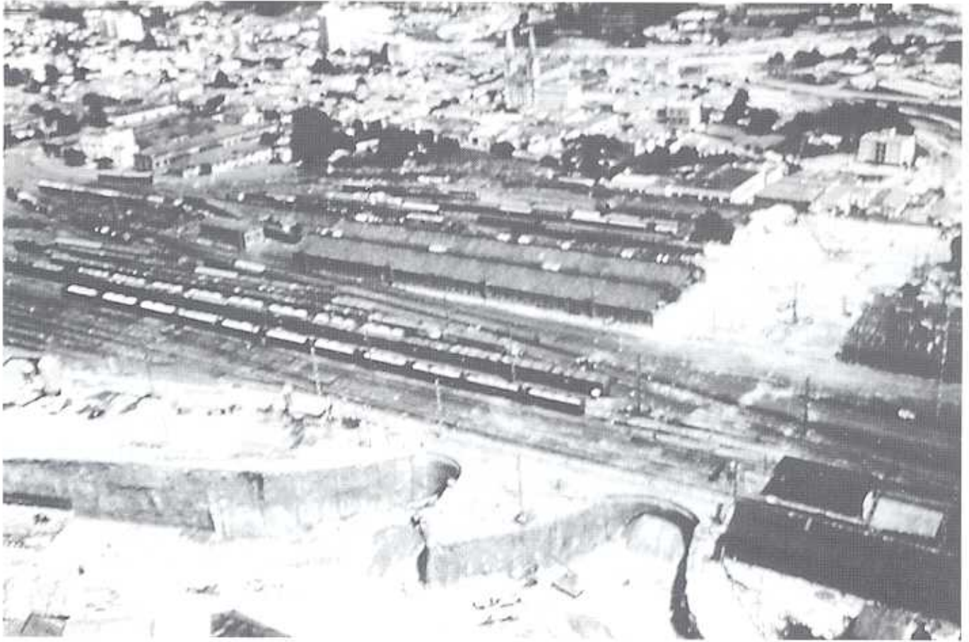
Fig. 32. Underpass built in sand without interrupting rail traffic in Campinas (Brazil) using near-horizontal jet-grouting techniques
