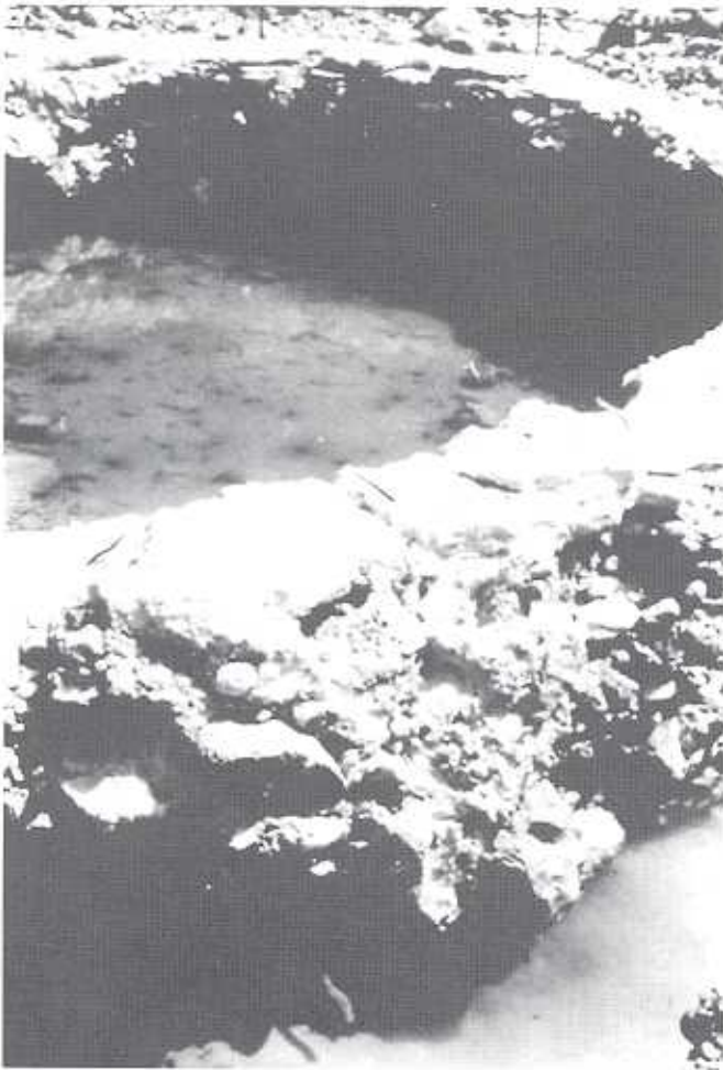
Fig. 25. Caissons under groundwater built using jet-grouting (railway bridge over the Fella River, Italy)
